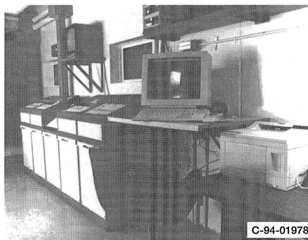
Figure 7.—Control room consoles.
