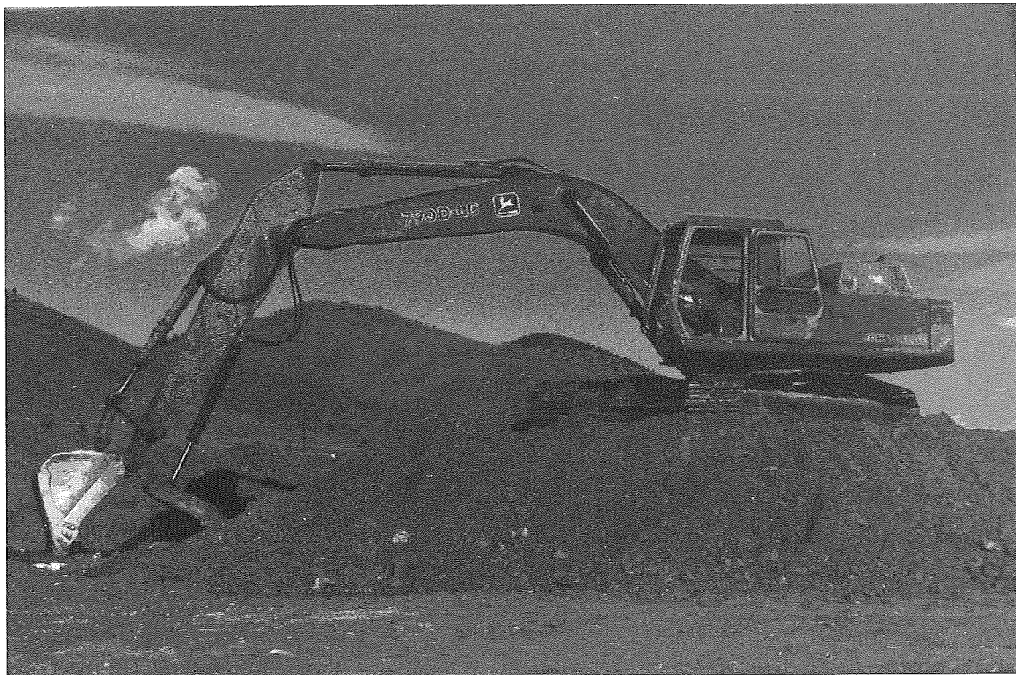
Figure 16. A small hydraulic shovel with a special gripping attachment on the bucket. Note the ability to dig below grade.
