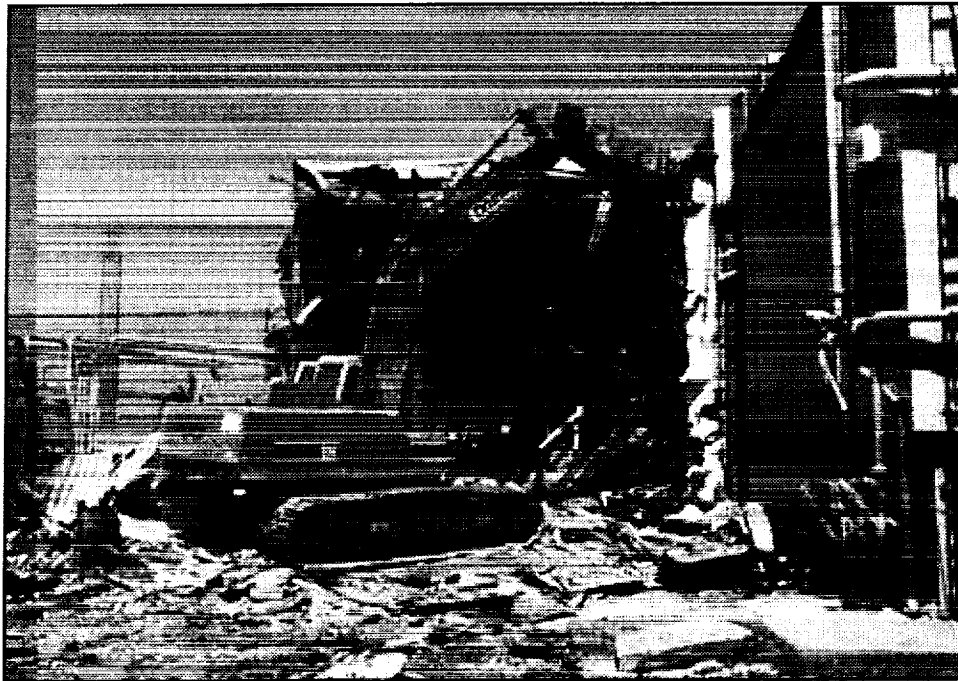
Figure 12. Demolition of Corner D and the original heat exchanger. Corner C is in the background. (C-99-1452)
