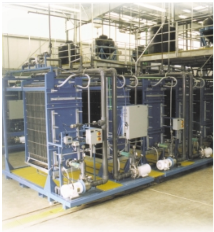
Osmotek, Inc.'s Direct Osmosis treatment system is being used to keep a landfill's surroundings clean.
