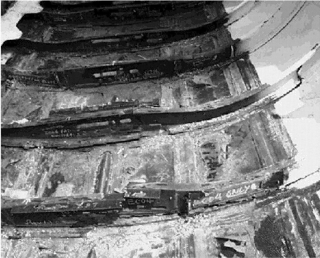
Figure C-4. Photograph showing interior damage and frame failure.
