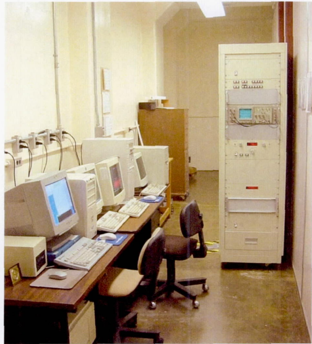
Figure 10 - Operations Area for the Compact Range Facility.
