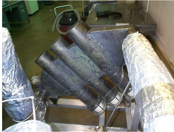
FIGURE 5. Gas Heater Assembly Before Insulation.
