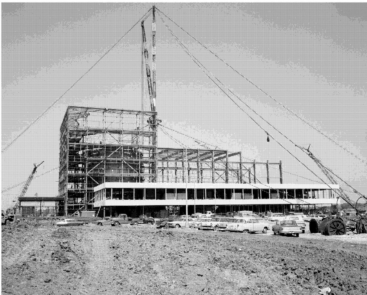
Construction March 1964 – Chamber A is visible to the left, administrative wing is in front of high bay.
