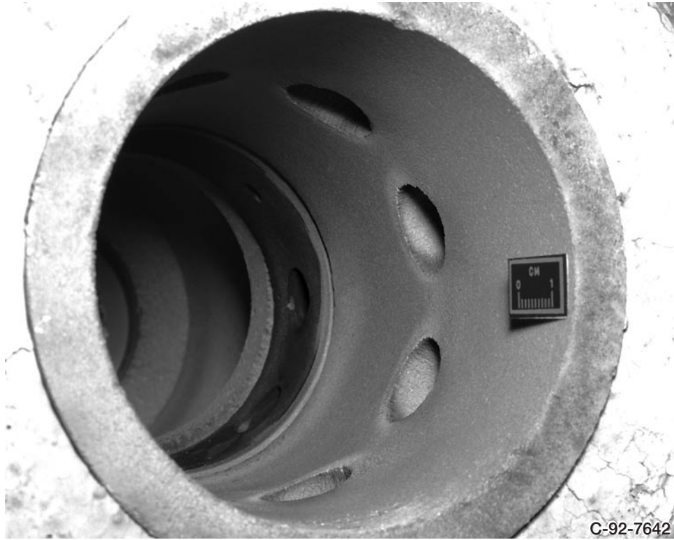
Figure 4.—Quick mixing module with castable liner.
