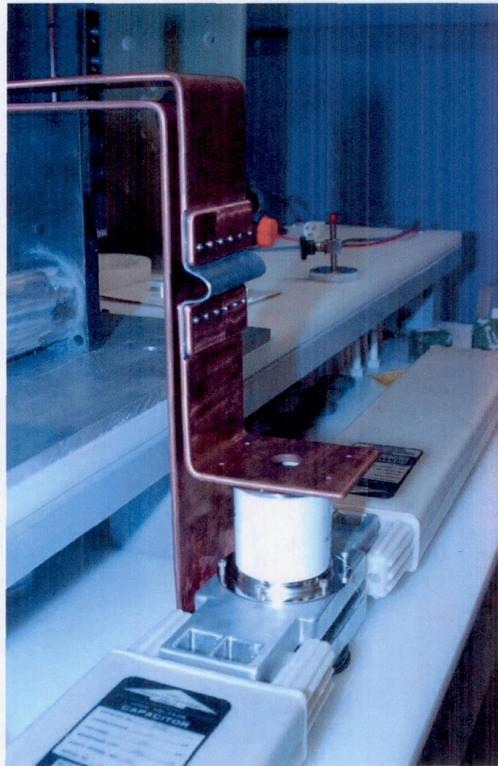
Capacitors, Switch and Bus
