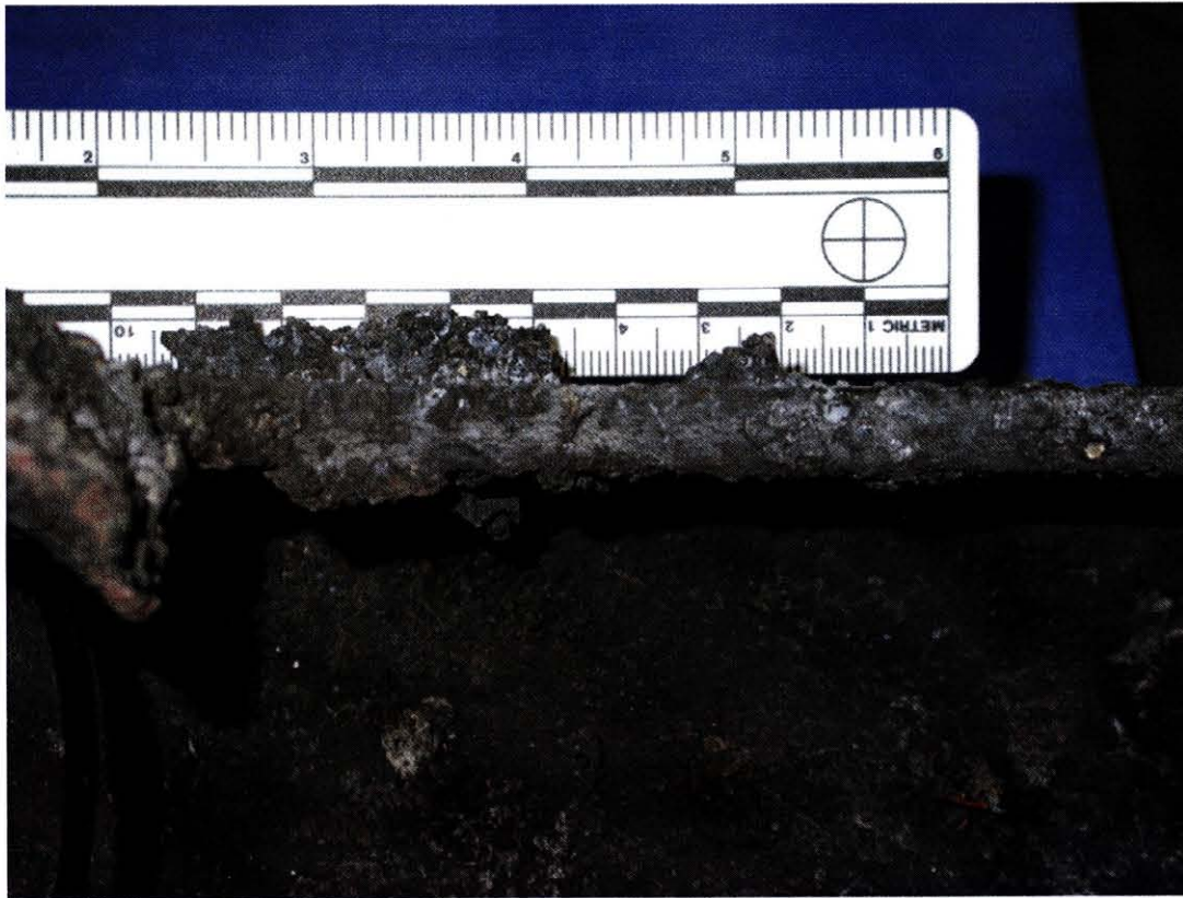
Figure 32: Slag Deposits on Upper Edge of Panel 8 on the RCC Side of the Vent.
