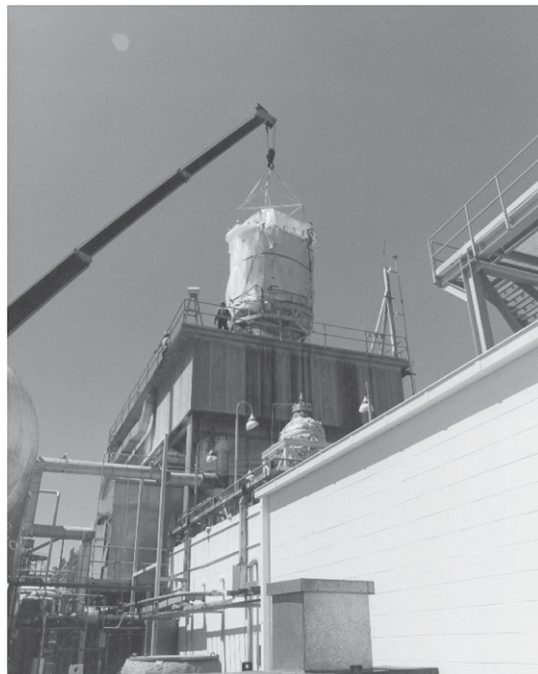
Figure 46. MHTB installation in test stand 300 vacuum chamber.
