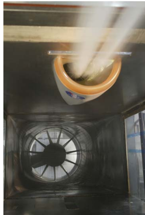
Figure 6a. Front view of inlet. BART tunnel fan also visible in background.
