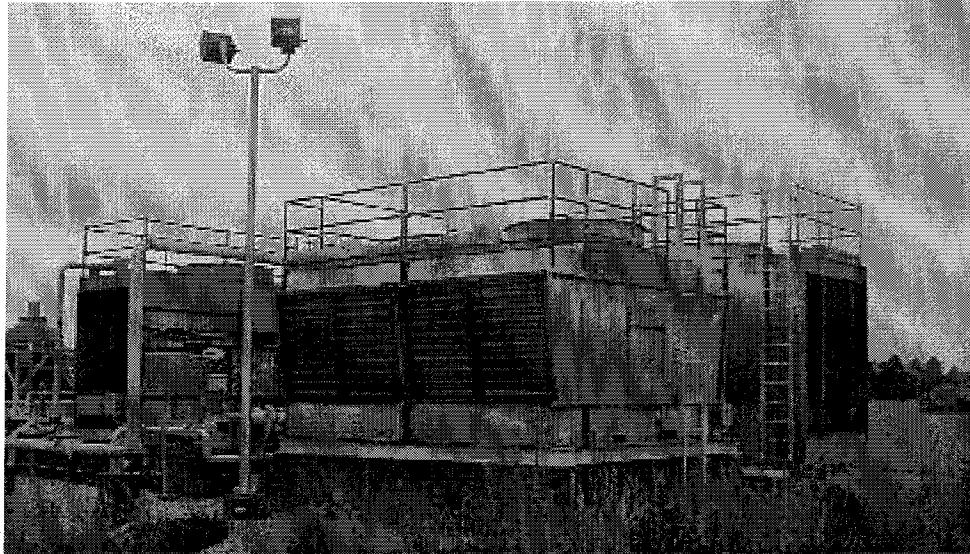
Cooling Water Towers at HPGF
