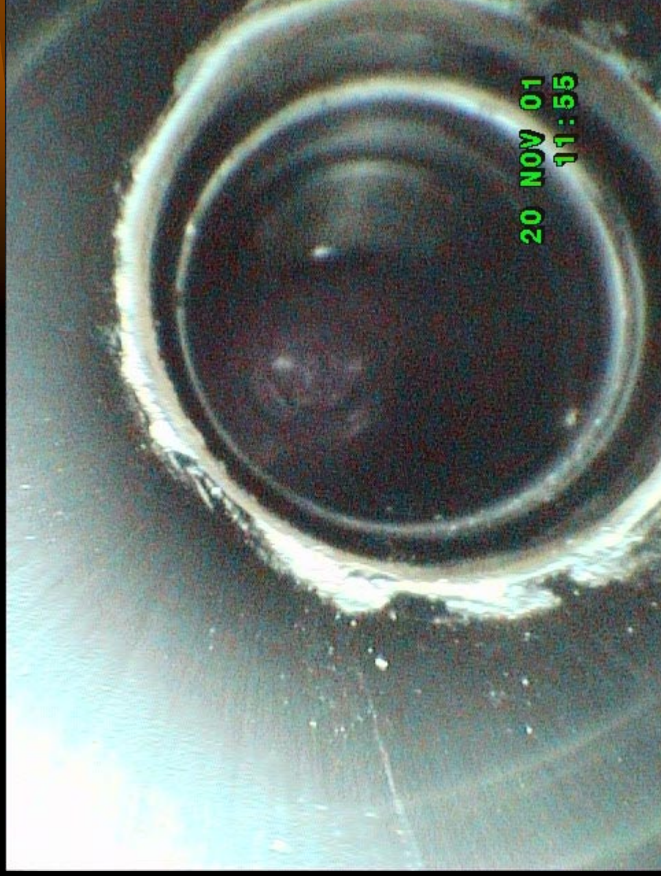
Figure 3. More damage from not removing a plug
