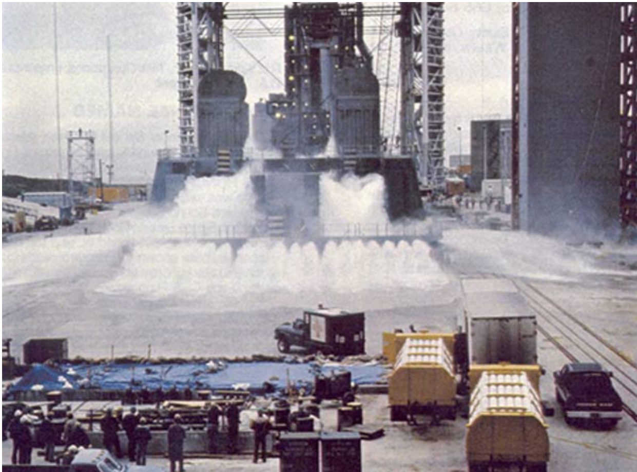
Figure 1. Original STS Deluge System Test (circa 1985)
