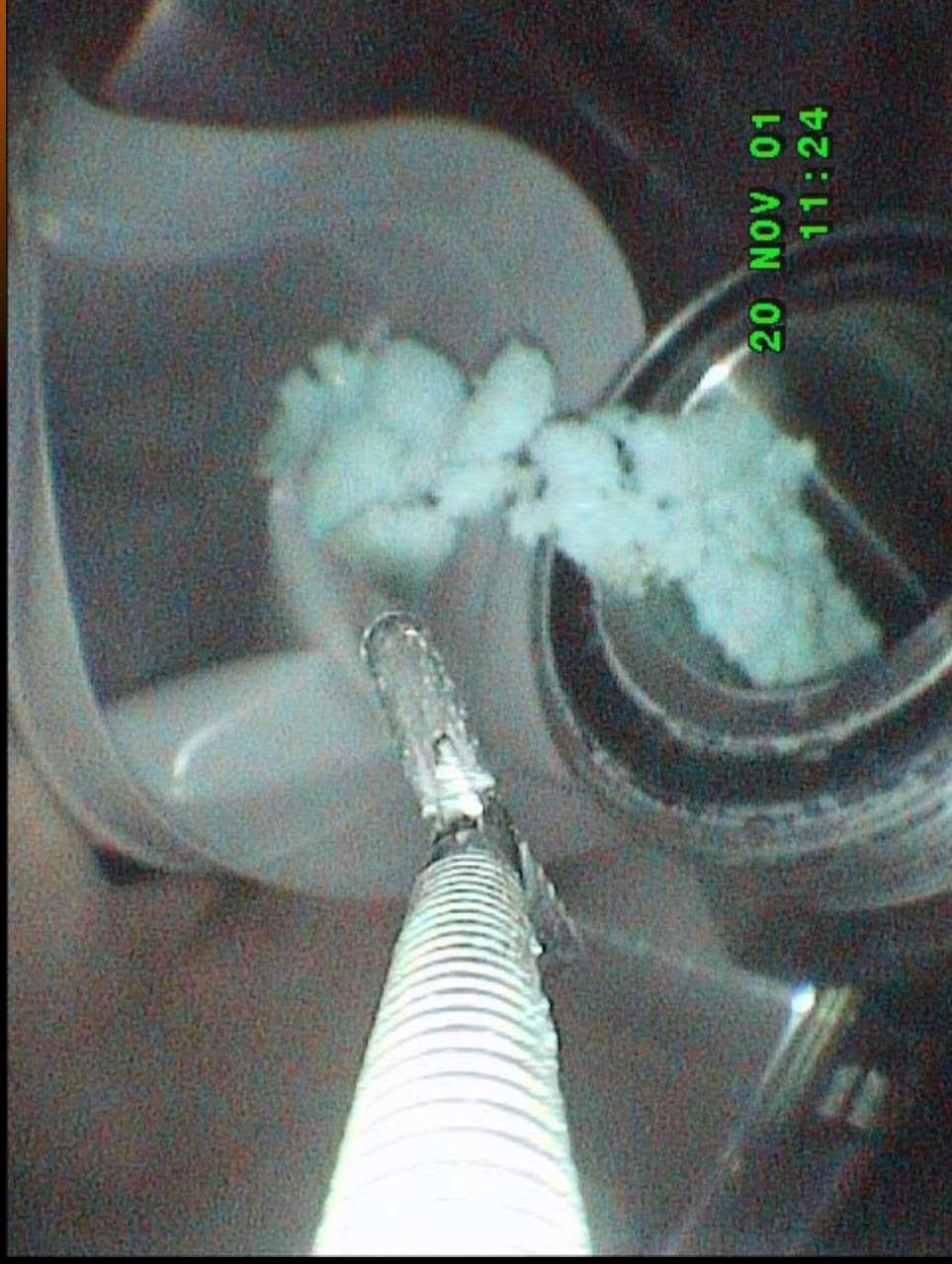
Figure 2. Damage from not removing a plug
