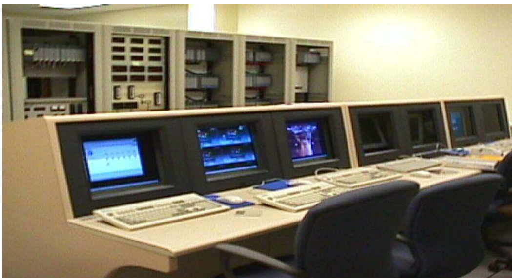
Figure 14. DACS Laboratory Control System Area.
