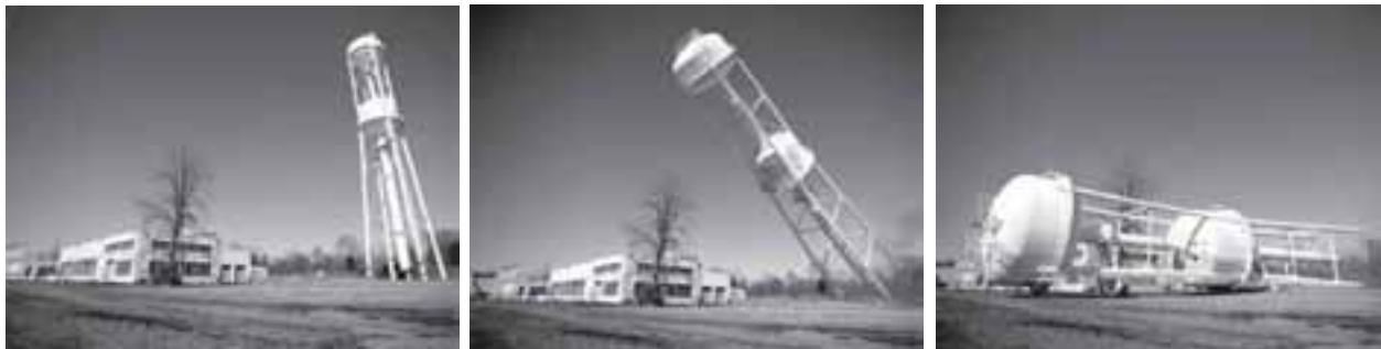
Image 127: Despite the fact that decommissioning work had been on-going since 2001, the felling of the 193-foot-tall double water tower was one of the first external signs that the Plum Brook reactor was being dismantled. The tower stood adjacent to the Reactor Facility from 1959 until its demolition in October 15, 2003. Workers placed explosive charges on the legs of the tower to collapse it in a controlled manner. The felled tower was then cut into pieces and shipped offsite for disposal. (NASA C-2004-742), (NASA C-2004-743), (NASA C-2004-744), (NASA C-2004-745)
