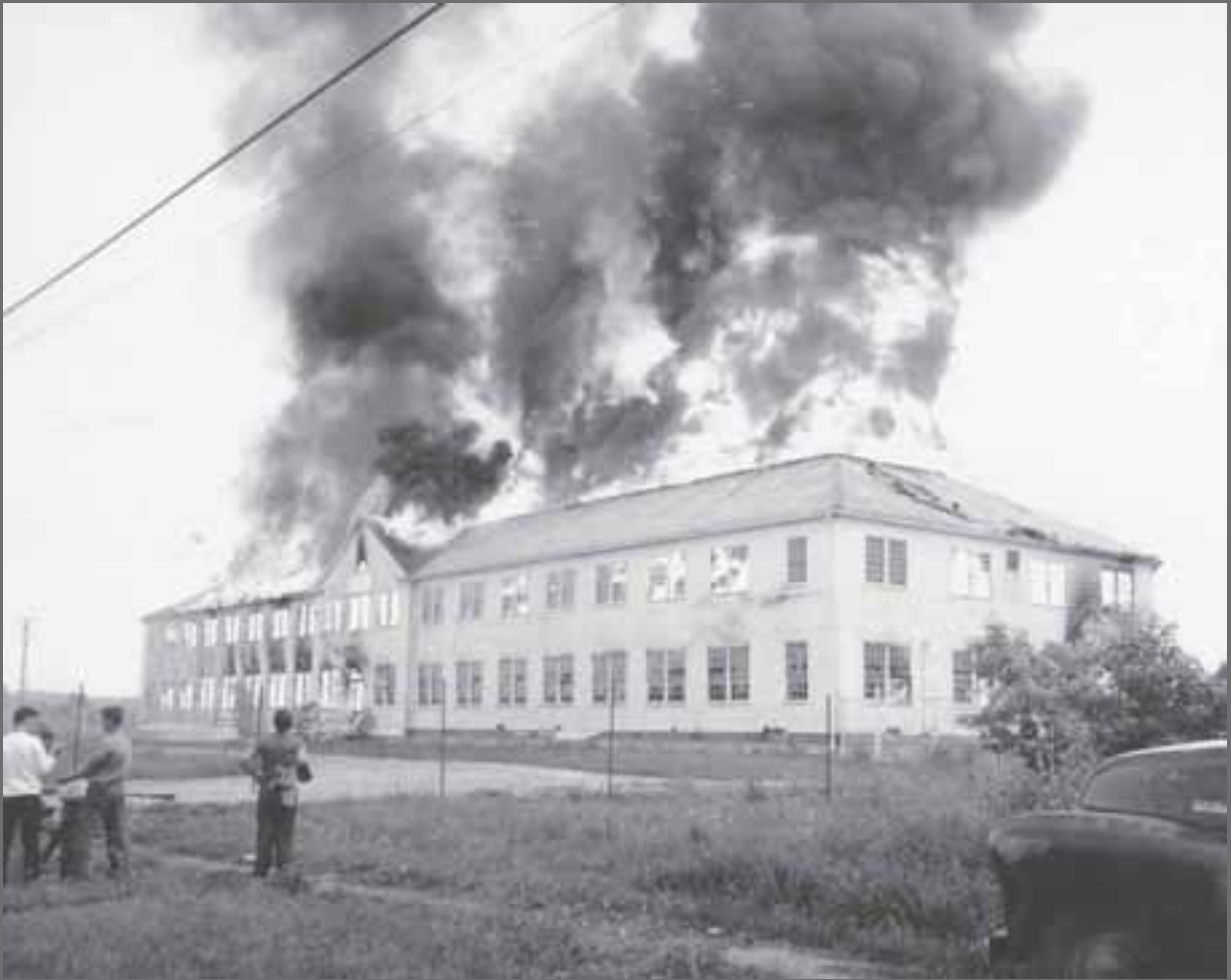
Image 40: Controlled fire to demolish unwanted Ordnance Works structure. Upon taking possession of Plum Brook, the NACA inventoried all the Ordnance Works structures and decided to retain forty-one of them, demolishing over 600 other buildings. In addition, three TNT areas and underground waste disposal lines had to be destroyed and decontaminated. (NASA C-2003-829)
