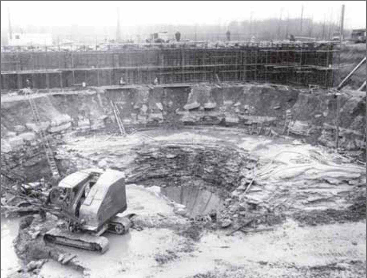
Image 42: The Plum Brook Reactor Facility construction began when crews excavated a hole in the ground for the pressure tank. The tank extended approximately thirty-two feet under ground. The steel containment vessel, which was more than 100 feet high (fifty-five feet above grade and fifty-six feet below grade), surrounded the reactor tank area and the surrounding quadrants and canals. It was designed to prevent any radioactivity from being released if an accident were to occur in the reactor. This safety precaution was essential because of the nearby communities. Many other large reactors did not have such safety features. For example, the Materials Test Reactor in Idaho Falls had no shield because small amounts of contamination could be released into the atmosphere without endangering the public. (1958–60) (NASA C–2003–830)
