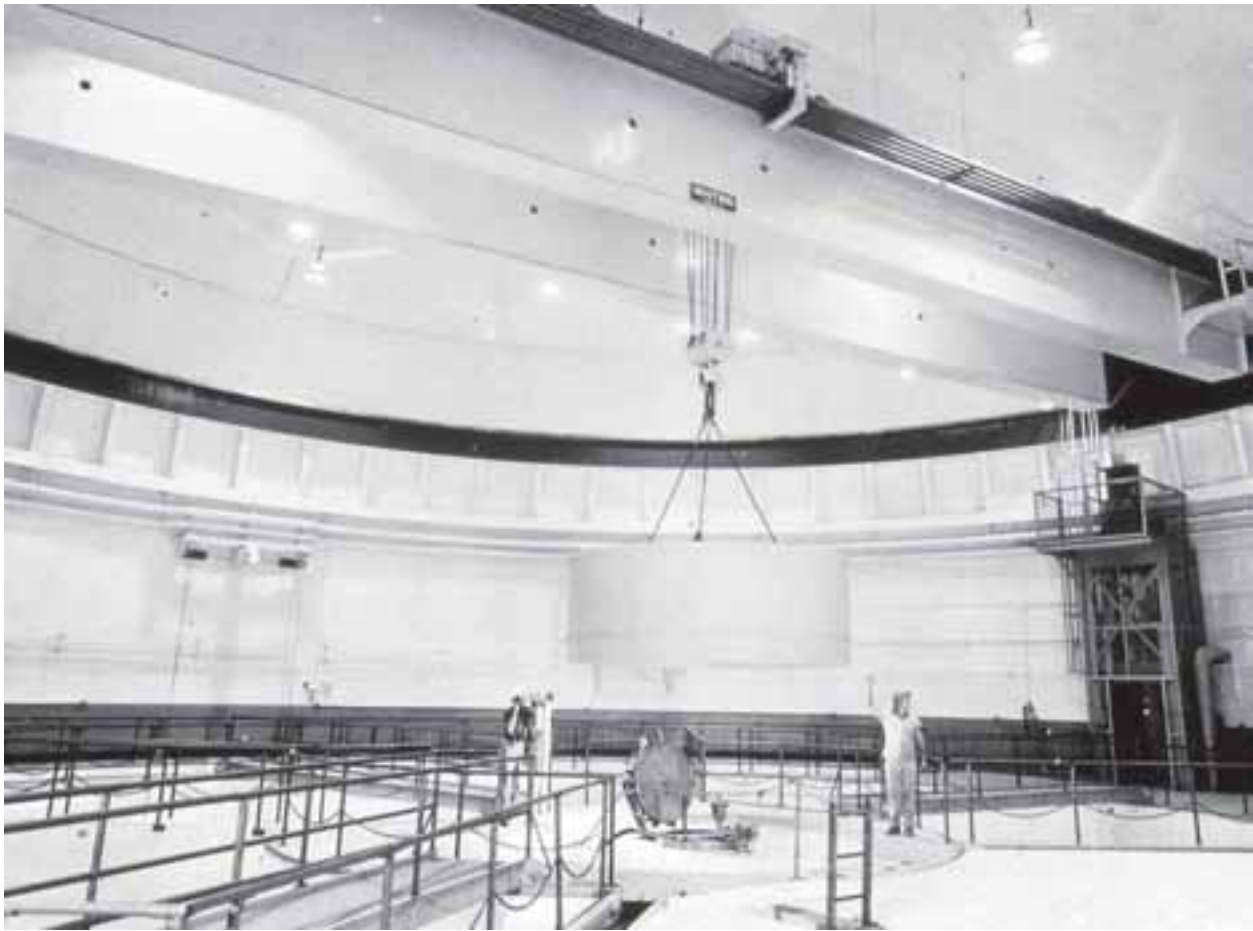
Image 64: Two men standing on the lily pad guide a crane to remove the third of three large, white, twenty-ton shrapnel shields that nest over the pressure tank. The shields were then stacked off to the side until it was time to reposition them on top of the pressure tank. Since the support beams could rotate 365 degrees, the overhead crane could reach any location in the containment vessel. The pressure tank hatch is open. (1959) (NASA CS-18228)
