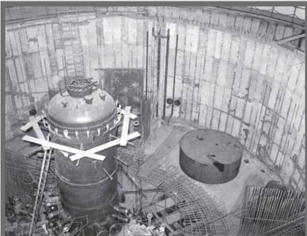
Image 49: The pressure tank in place inside the containment vessel. (NASA C-2003-836)
