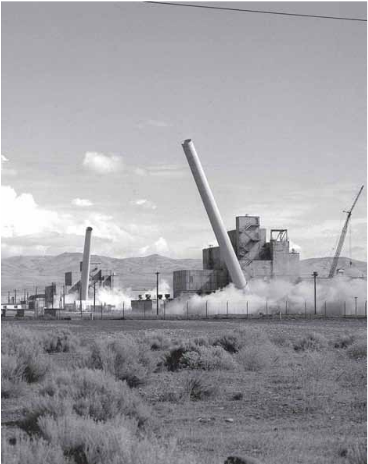
Image 122: Two stacks are felled simultaneously during the decommissioning of the Hanford reactor. In recent years, several other reactors besides Plum Brook have been decommissioned. Successful decommissioning projects include the Watertown Arsenal, Shoreham, the Saxton Nuclear Experimental Corporation, Argonne, Pathfinder, Elk River, Fort St. Vrain, Shippingport Nuclear Power Station, and Trojan. (1977) (Department of Energy Photo 1001138)
