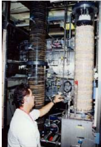
Biological Water Recovery System
