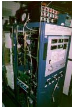
Carbon Dioxide Removal System
