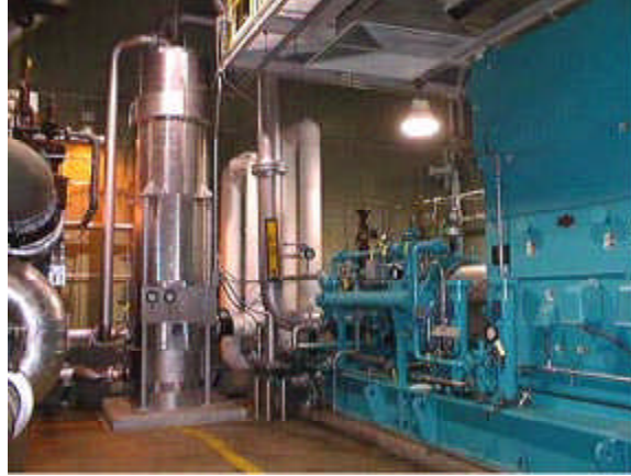
Compressor C-18 with electric drive motor and auxiliary systems.
