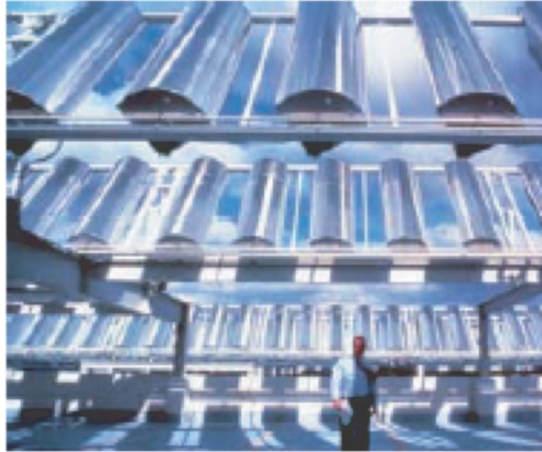
Figure 8.—A 300-kilowatt linear concentrator system (courtesy of the National Renewable Energy laboratory).
