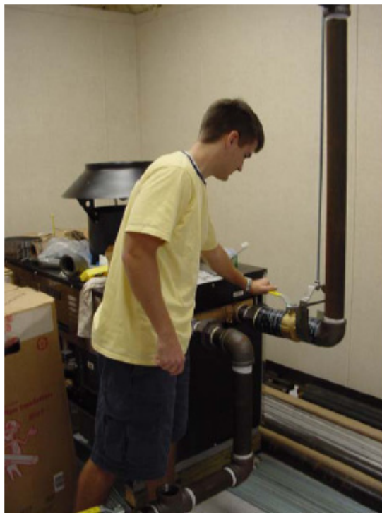
Figure 7.—Heating Hot Water Boiler.
