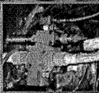
Pressure Transducer and Fire Valves
