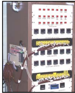
Completed Heater Controls
