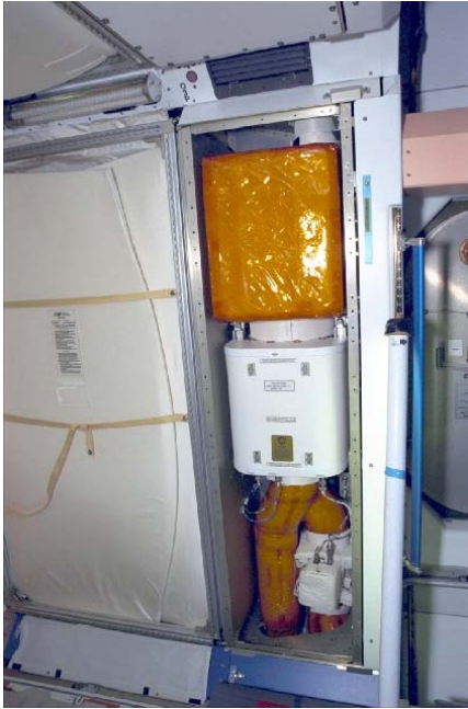
Node 1 Inlet ORU, Cabin Diffuser, and the Node 1 VAVDA
