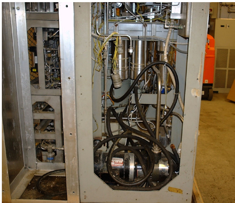
Figure 2.9.—Electrolyzer stack power cables and data acquisition cable bundle.
