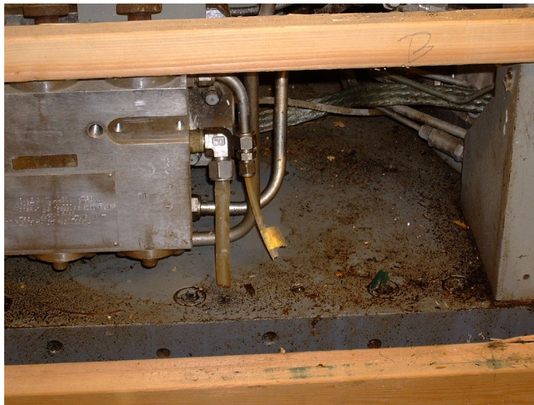
Figure 2.11.—Base of the OGP next to the distilled water feed pump.
