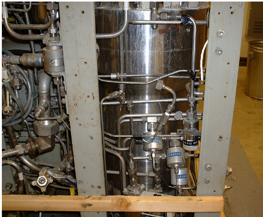
Figure 2.7.—Unconnected process lines in front of the electrolyzer stack pressure vessel.
