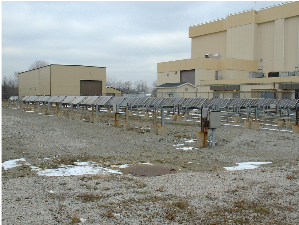
Figure 4.2.—Present array field.
