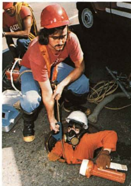
While one technician mans a safety line, another descends into a sewer to position the waterflow monitoring equipment. The system helps locate pollution-causing sewer leaks.
