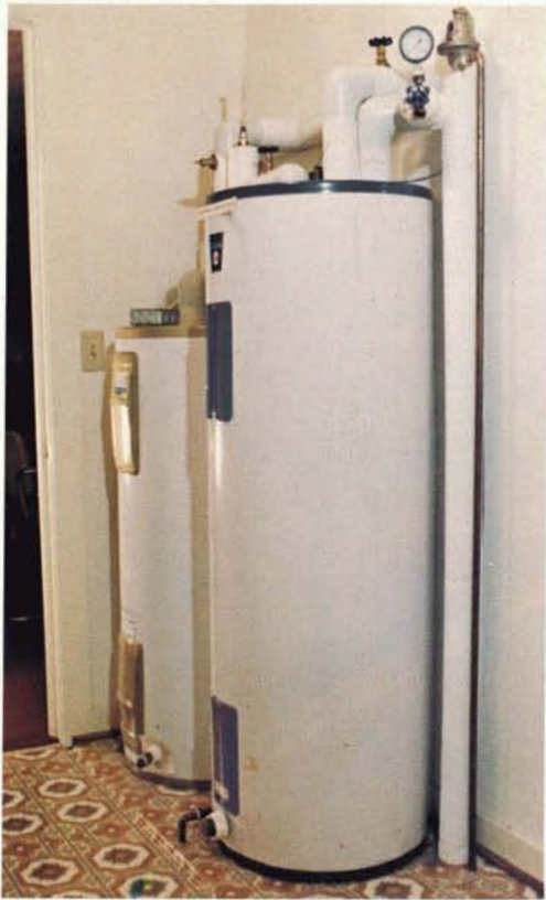
These two tanks make up a unique Tech House domestic hot water system. Water in one tank is "preheated" by solar energy, then fed into the other tank where a conventional electric heater further raises the temperature if necessary. Preheating takes care of 80 percent of the hot water energy requirement.
