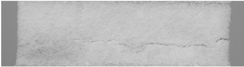
a. Initial stage of cracking.
