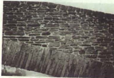
Fig. 1.3 Voussoirs and parapet at Pontypridd (photographed by Ted Riddock, reproduced by permission of Cambridge University Press).
