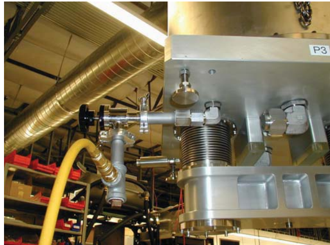
Figure 14 Low-leakage vacuum valve used in leak rate tests
