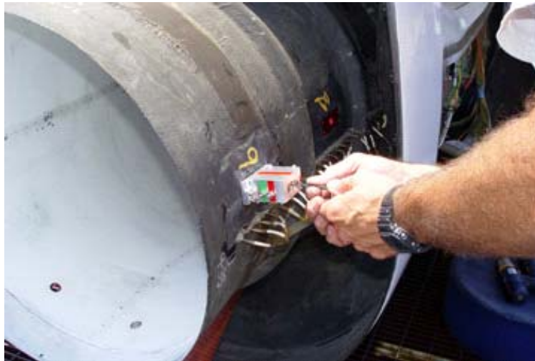
Fig. 3-6 Mounting of pressure module on the outer side of an inlet wall.
