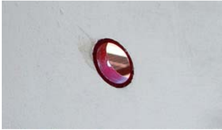
Fig. 3-5 Access port in the left inlet wall (view from inside of inlet duct).
