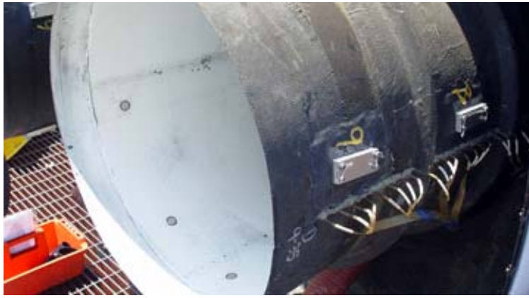
Fig. 3-8 Unused access ports closed with wall plugs.
