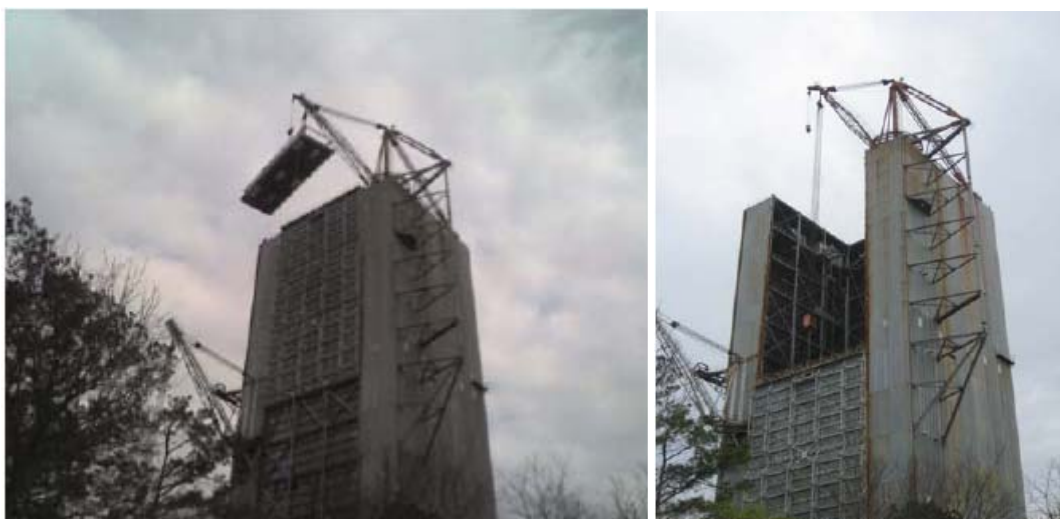
Figure 3. The roof panels were removed and the main door was lowered (opened) on Test Stand 4550 for the first time in 29 years this past April.
