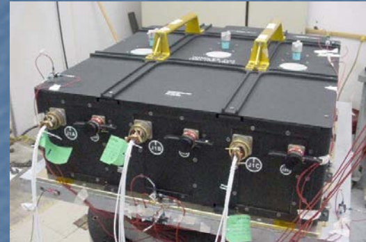
Replace the 3 batteries
