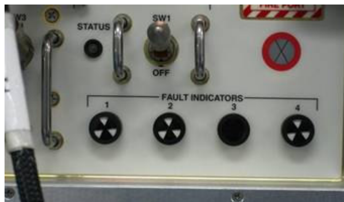
Figure 38. Example Fault Indication After an Automatic Shutdown
