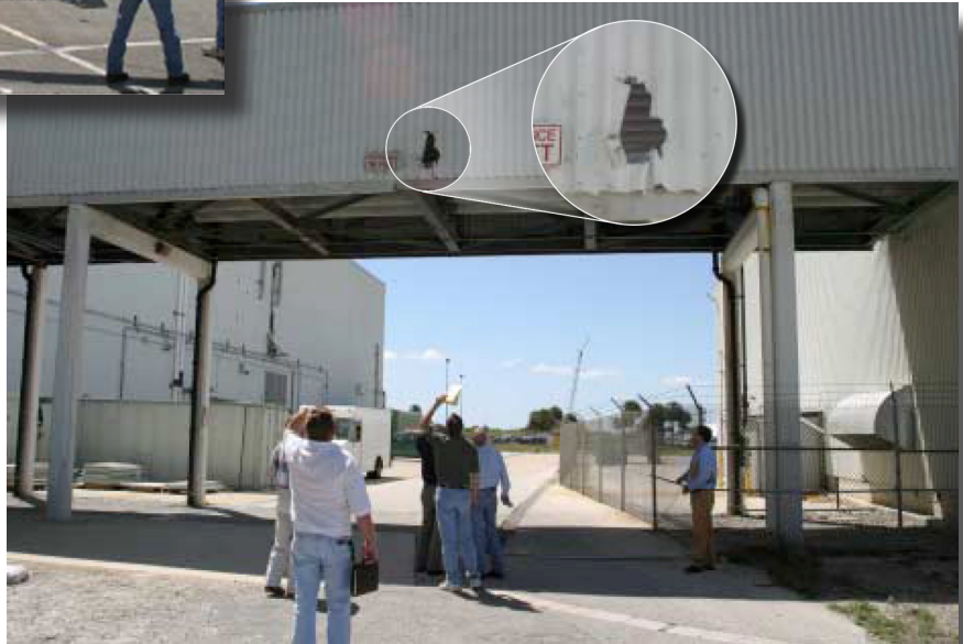
Location and close-up of damage to the crossover between the KSC Vehicle Assembly Building and a utility annex.
