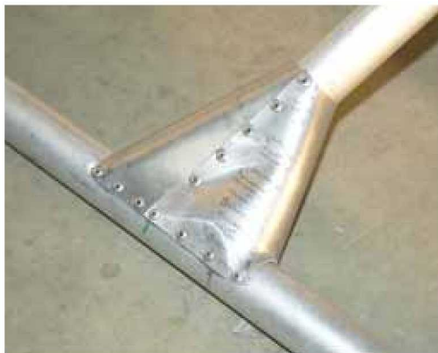
(a) Photo depicting saddle buckling.
