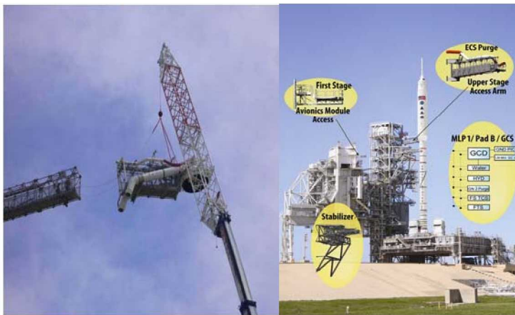
Figure 4. Gaseous oxygen arm being removed (left) and artist's concept (right) depicting hardware added to LC 39B for Ares I-X.
