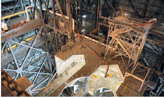
Figure 3. Platform C was removed from the VAB's High Bay 3 (top) and other platforms were added (bottom) to give ground operations staff access to the Ares I-X interstage segment.
