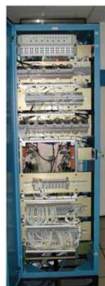
Figure 5. The GC3 rack installed in the Mobile Launcher Platform also is used to control Atlas V.
