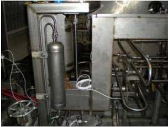
Cable tray providing protection from heat/NaK
