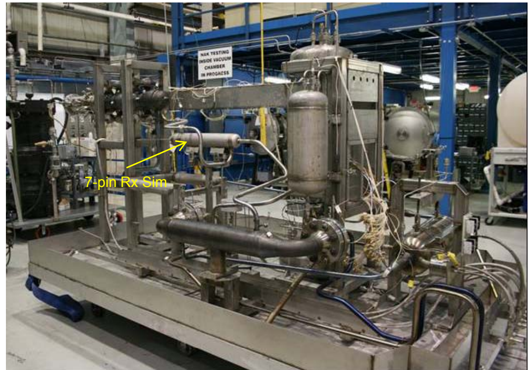
7 Pin Rx Core Sim installed in FSP-PTC
