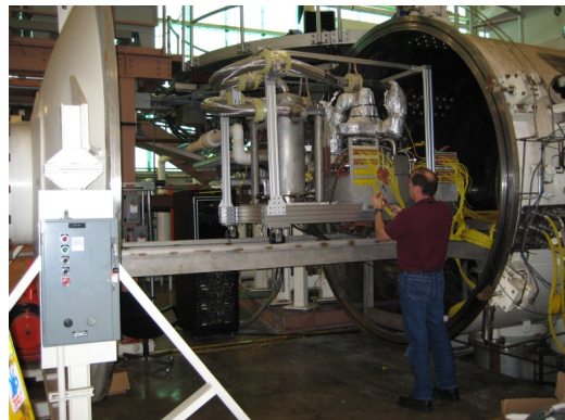
Figure 6.—Direct drive gas Brayton test system.
