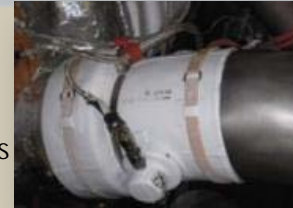
New Liquid Air Insulators
