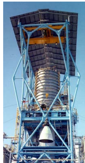
Figure 14. Apollo SPS Engine being Hoisted up to the J-3 Test Cell Capsule
