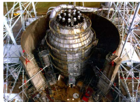
Figure 22. J-4 Test Chamber Capsule and LH 2 /Cold GHe HEX inside the Blast Wall
