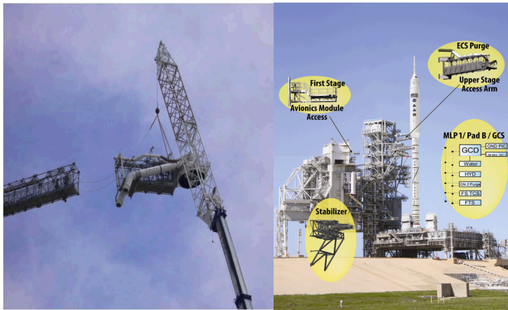
Figure 9. Gaseous oxygen arm being removed (left) and artist’s concept (right) depicting hardware added to LC 39B for Ares I-X.
