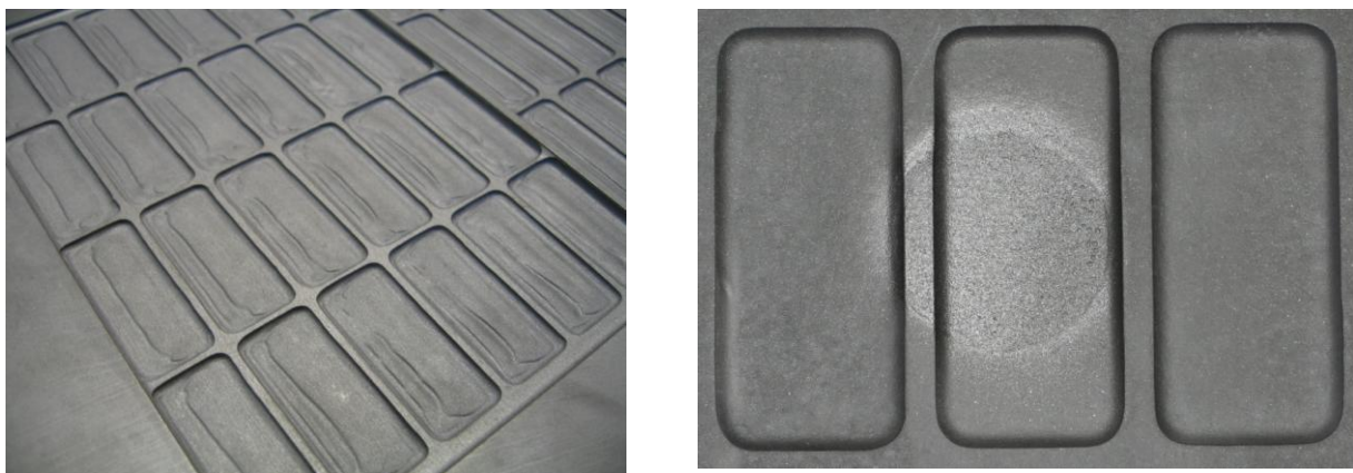
Figure 8. Thermal barrier coating panel showing 'ridging,' left, and test repair, right
