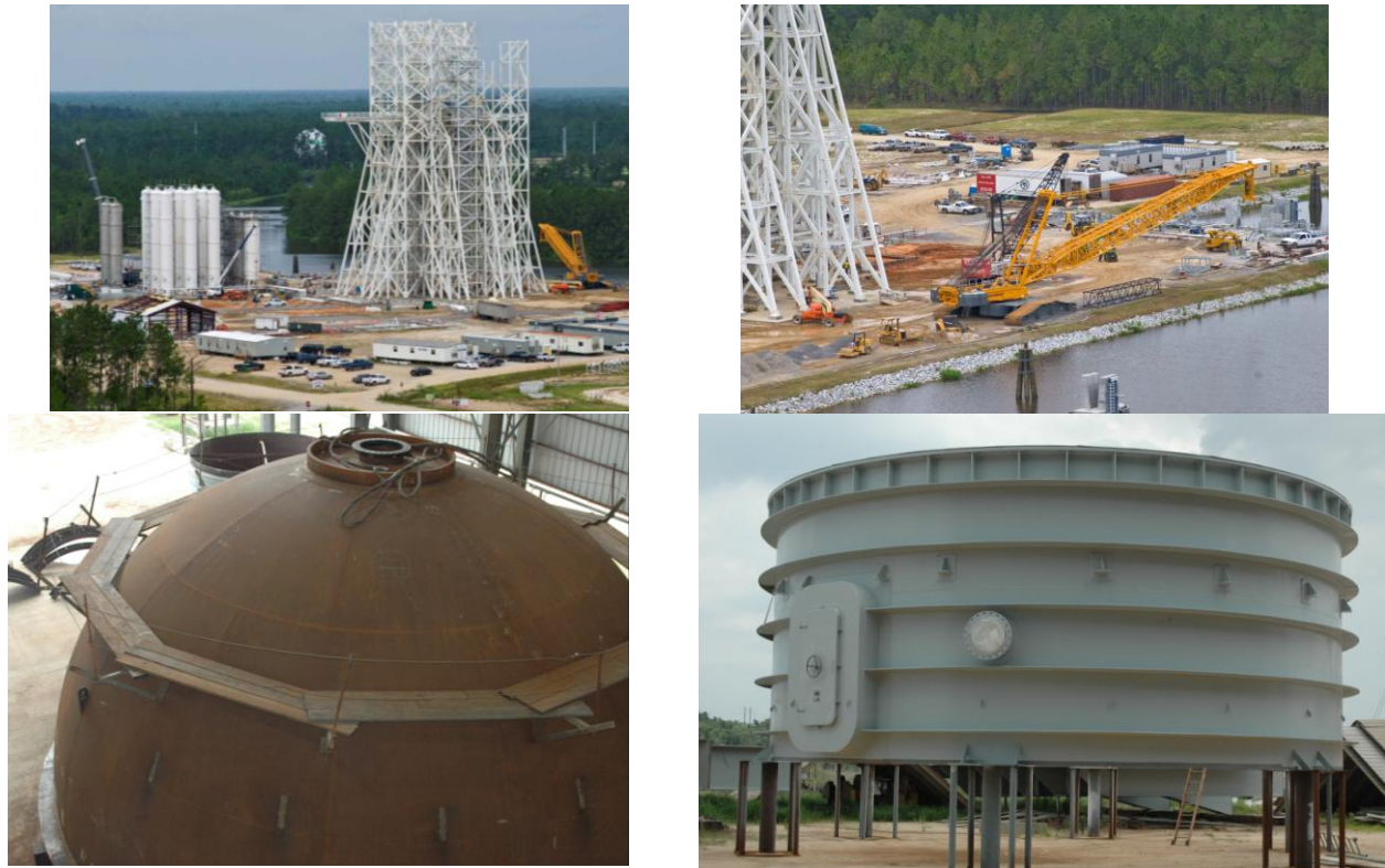
Figure 11. A3 test site, June 2010, clockwise from upper left: stand and IPA, water and LOX tanks; crane, test cell bottom section; and test cell dome
