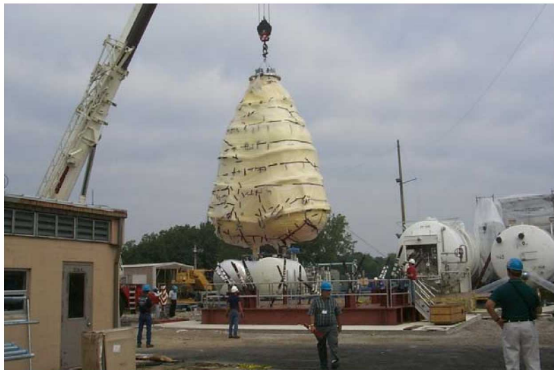
Figure 21. Installation of the STA Tank at the GRC South Forty Test Facility.
