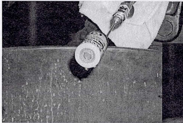
Epoxy on the vent
