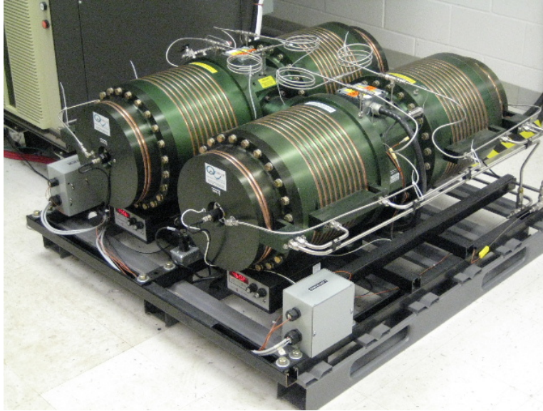
Figure 1.—Compressor alternator pairs as installed.
