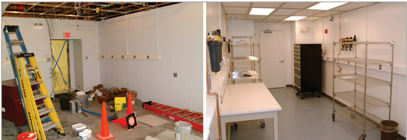
Two laboratories undergoing renovation: A laboratory in the middle of the renovation process (left) contrasted to a completed laboratory (right)—from chaos to order. In these laboratories, we will develop and test innovative technologies and build new instrumentation to enable future NASA solar and space physics missions.
