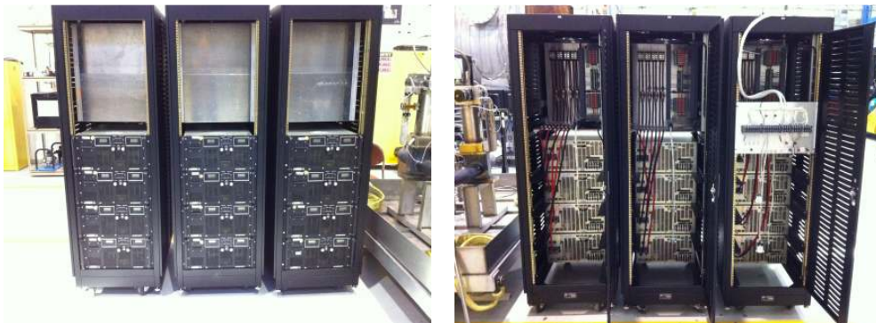
FIGURE 11. Power Distribution Racks.
