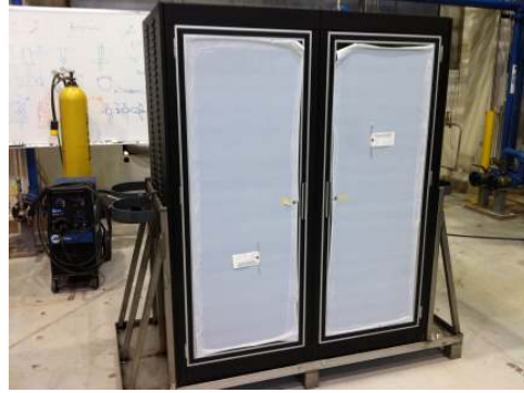
FIGURE 10. Gas System Racks.
