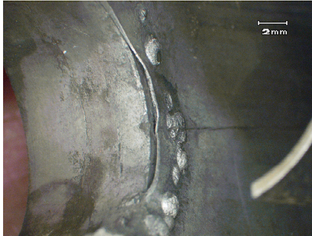
Figure 4.—Different view of the welding defects observed at the loop/outlet pipe joint. “metal bubbles” (nuggets) left from the welding process and open gap are visible.
