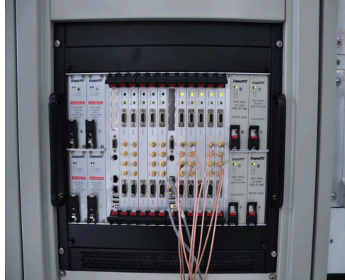
Figure 4. Two CDAS systems integrated into one box.
